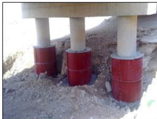
Figure 5: Treatment of damaged joint by RC Confined by Steel Casing (After Concrete Poured)
